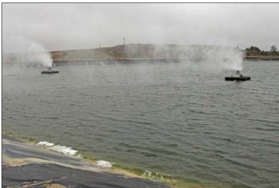
Waste water from the Wild Turkey system goes to evaporation ponds (Fig2).
